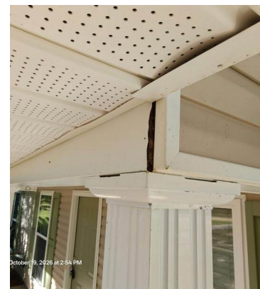
Kickout flashing missing
